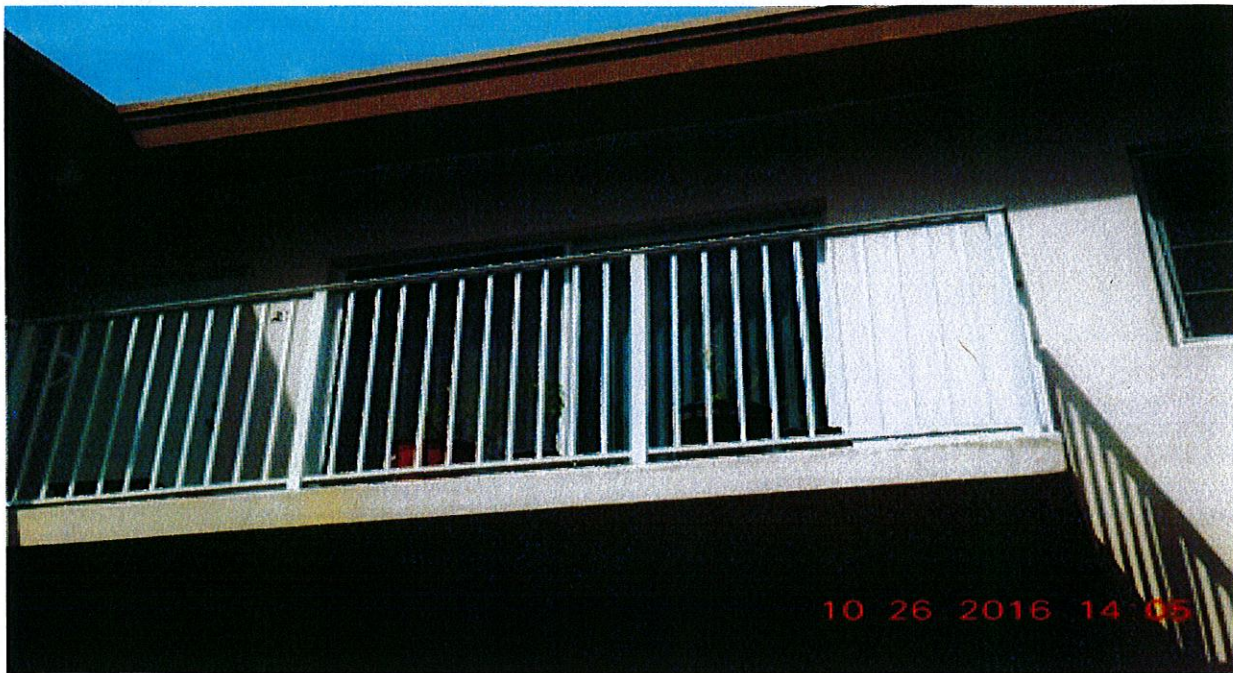
Unit #27- No violations observed. (14 of 16)
