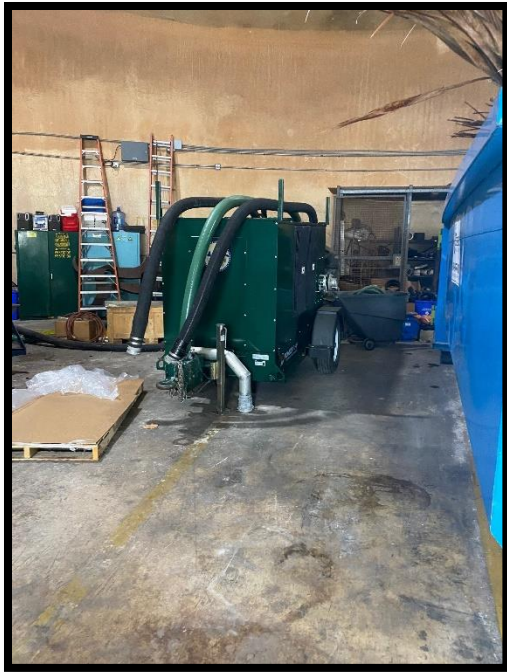
Figure 7: Temporary Sewer Pump
