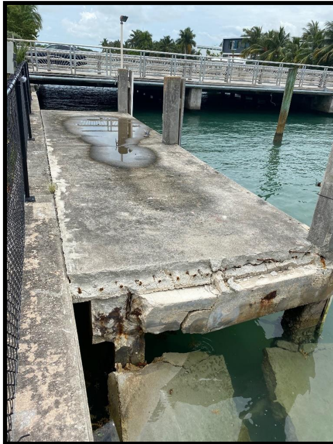
Figure 3: Existing seawall in critical condition and collapsed concrete dock
