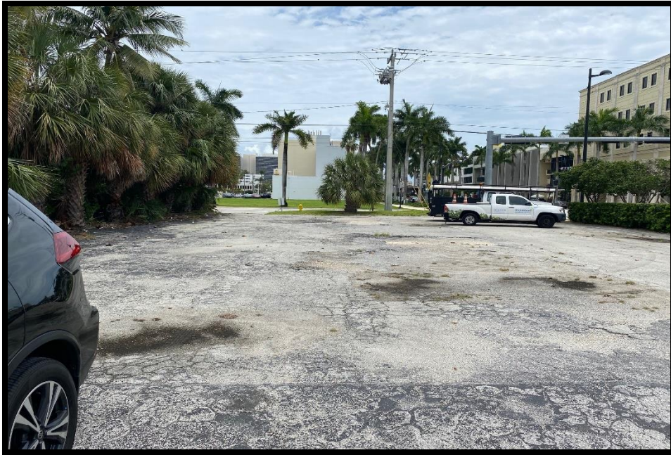
Figure 2: Existing Deteriorated Condition of the Lot
