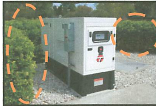
(2). Evergreen screening surrounds mechanical equipment on a minimum of three sides.
