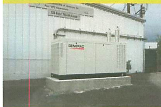
(above) Generac standby commercial generator without sound-proofing panel enclosure.
