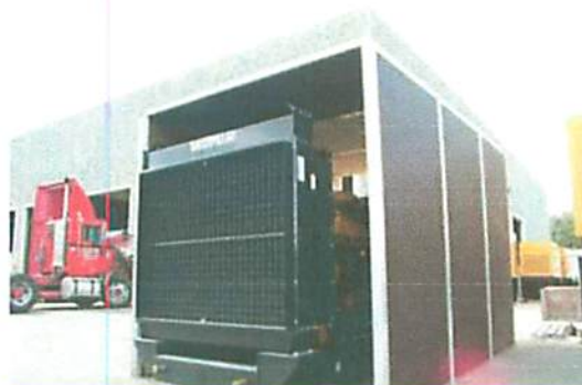
(above) Caterpillar commercial standby generator with sound-proofing panel enclosure.
