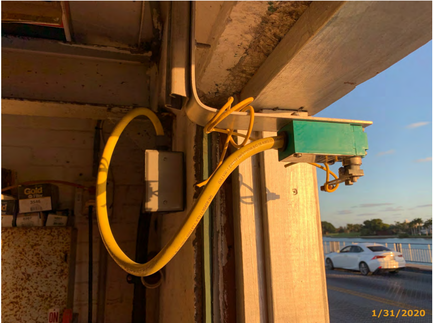
Photo 8574-E02 (Element/Env 8574/I: Control Console)
