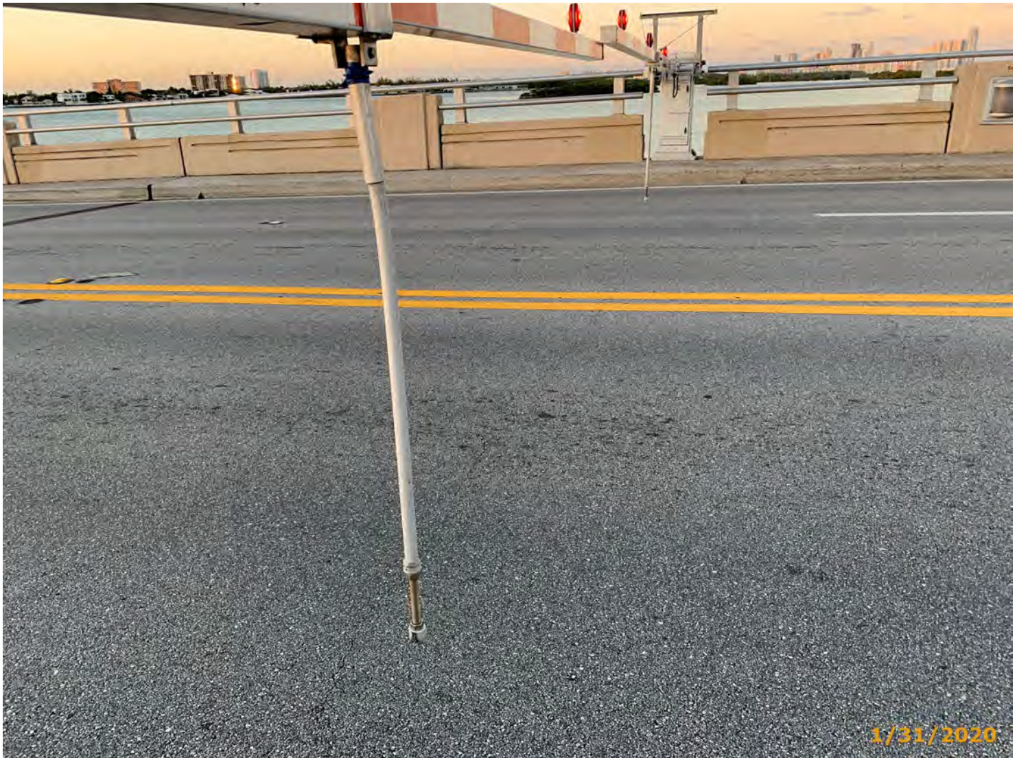
Photo 8591-E03 (Element/Env 8591/4: Warning Gates)
