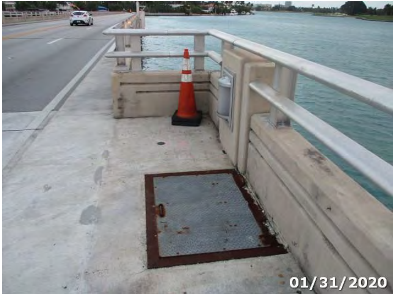
Photo 12-05 (Element/Env 12/4: Re Concrete Deck)
