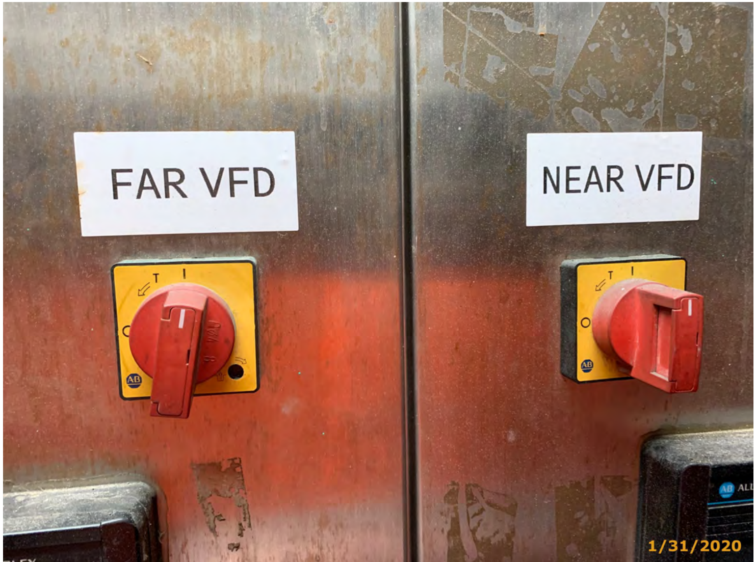
Photo 8546-E01 (Element/Env 8546/4: Span Drive Motors)
