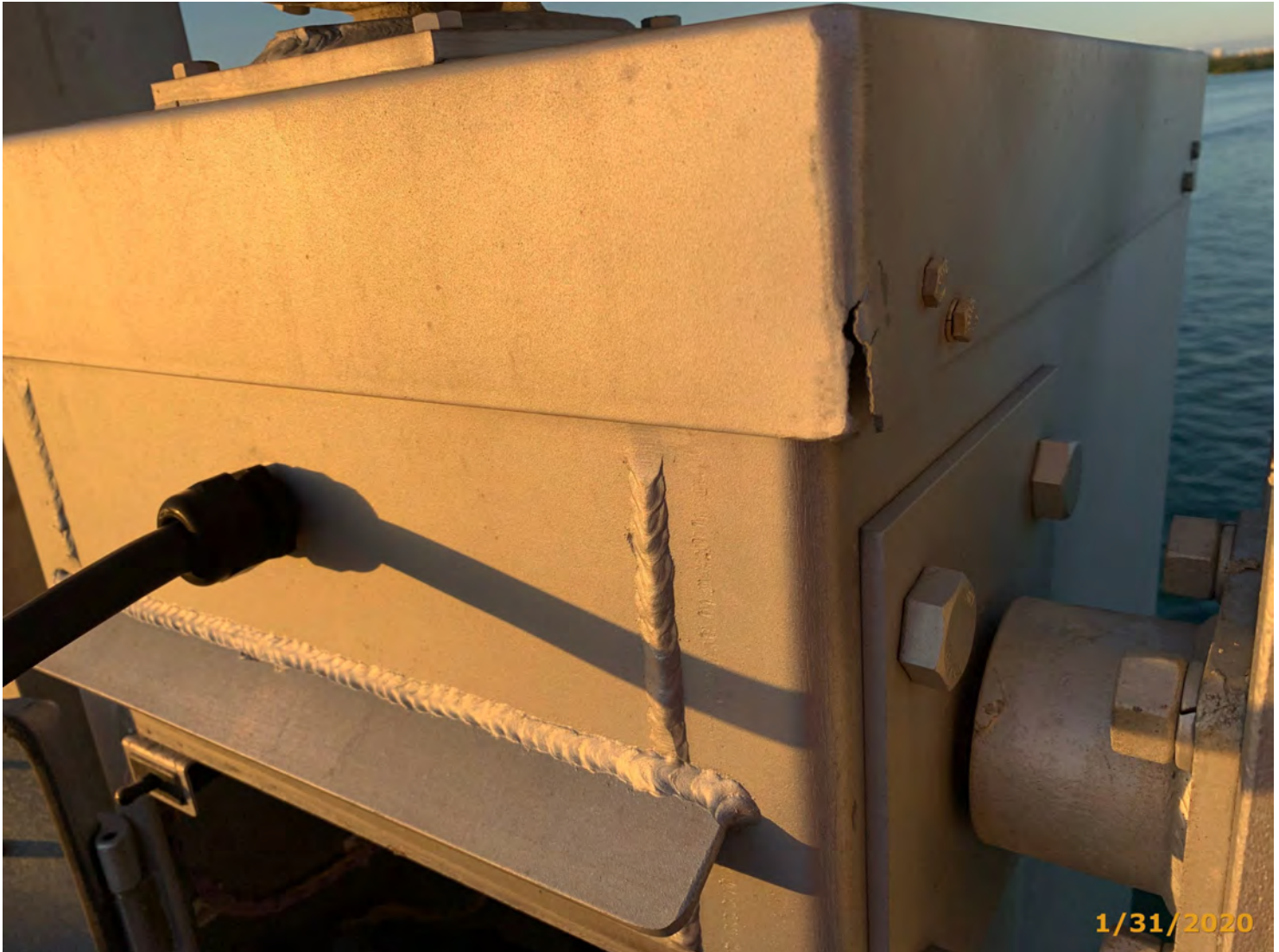
Photo 8591-E01 (Element/Env 8591/4: Warning Gates)
