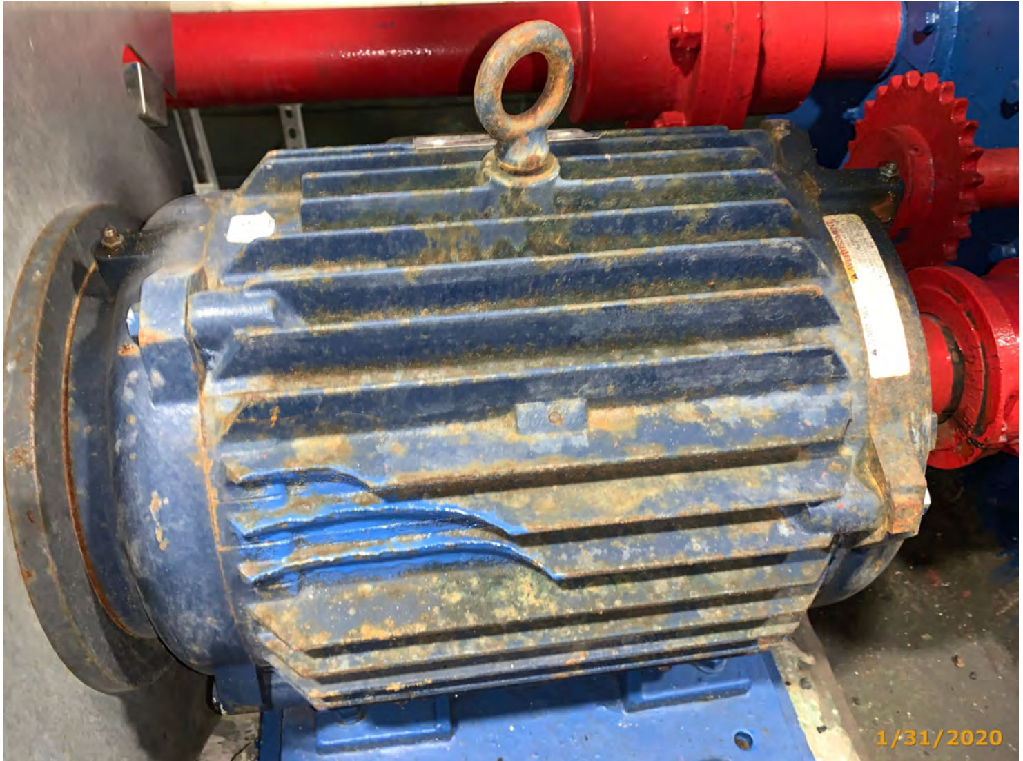
Photo 8546-E02 (Element/Env 8546/4: Span Drive Motors)
