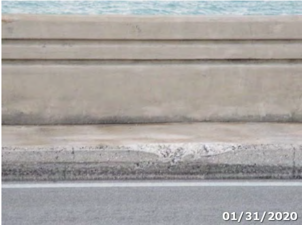
Photo 12-04 (Element/Env 12/4: Re Concrete Deck)
