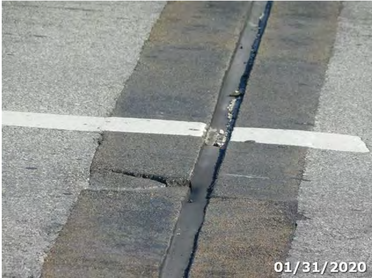
Photo 301-01 (Element/Env 301/4: Pourable Joint Seal)
