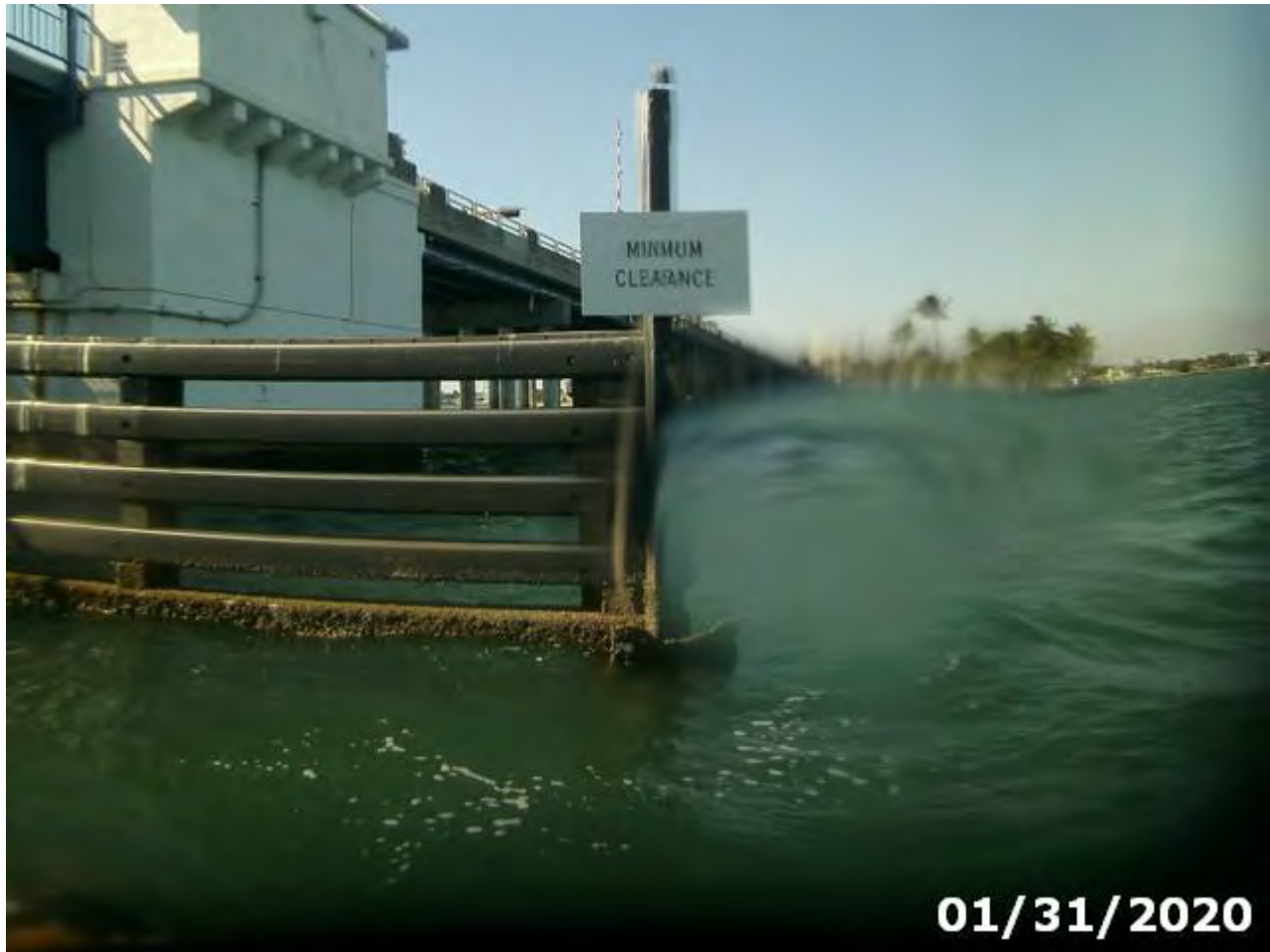
Photo 8390-02 (Element/Env 8390/4: Other Fender/Dolphin)
