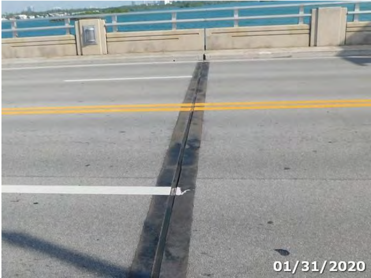
Photo 301-02 (Element/Env 301/4: Pourable Joint Seal)
