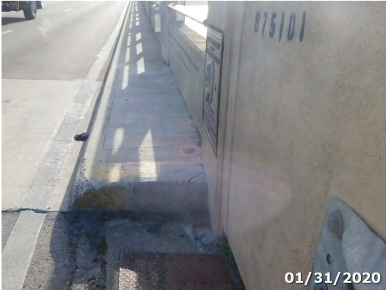
Photo 12-02 (Element/Env 12/4: Re Concrete Deck)
