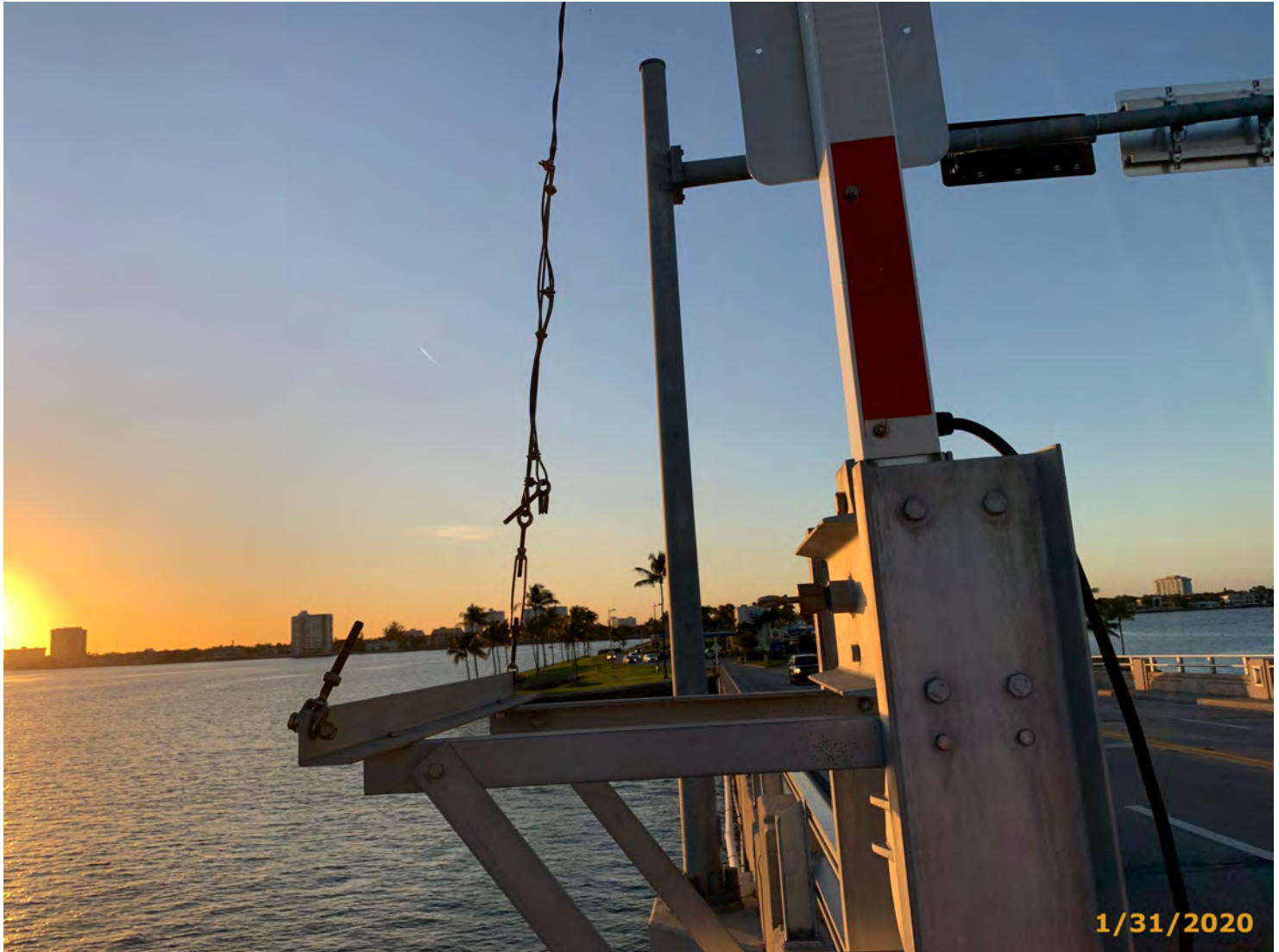
Photo 8591-E02 (Element/Env 8591/4: Warning Gates)
