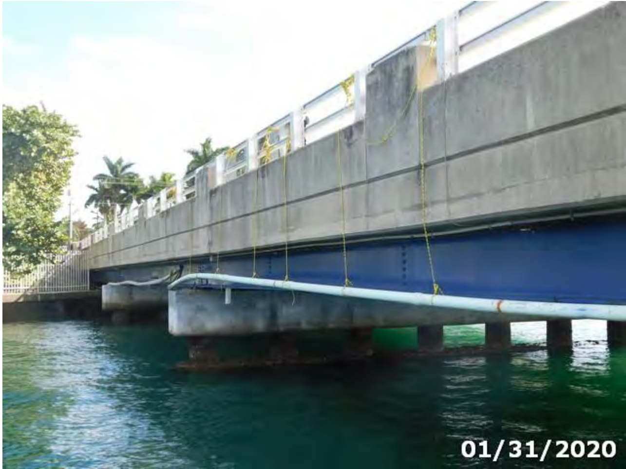
Photo 12-08 (Element/Env 12/4: Re Concrete Deck)
