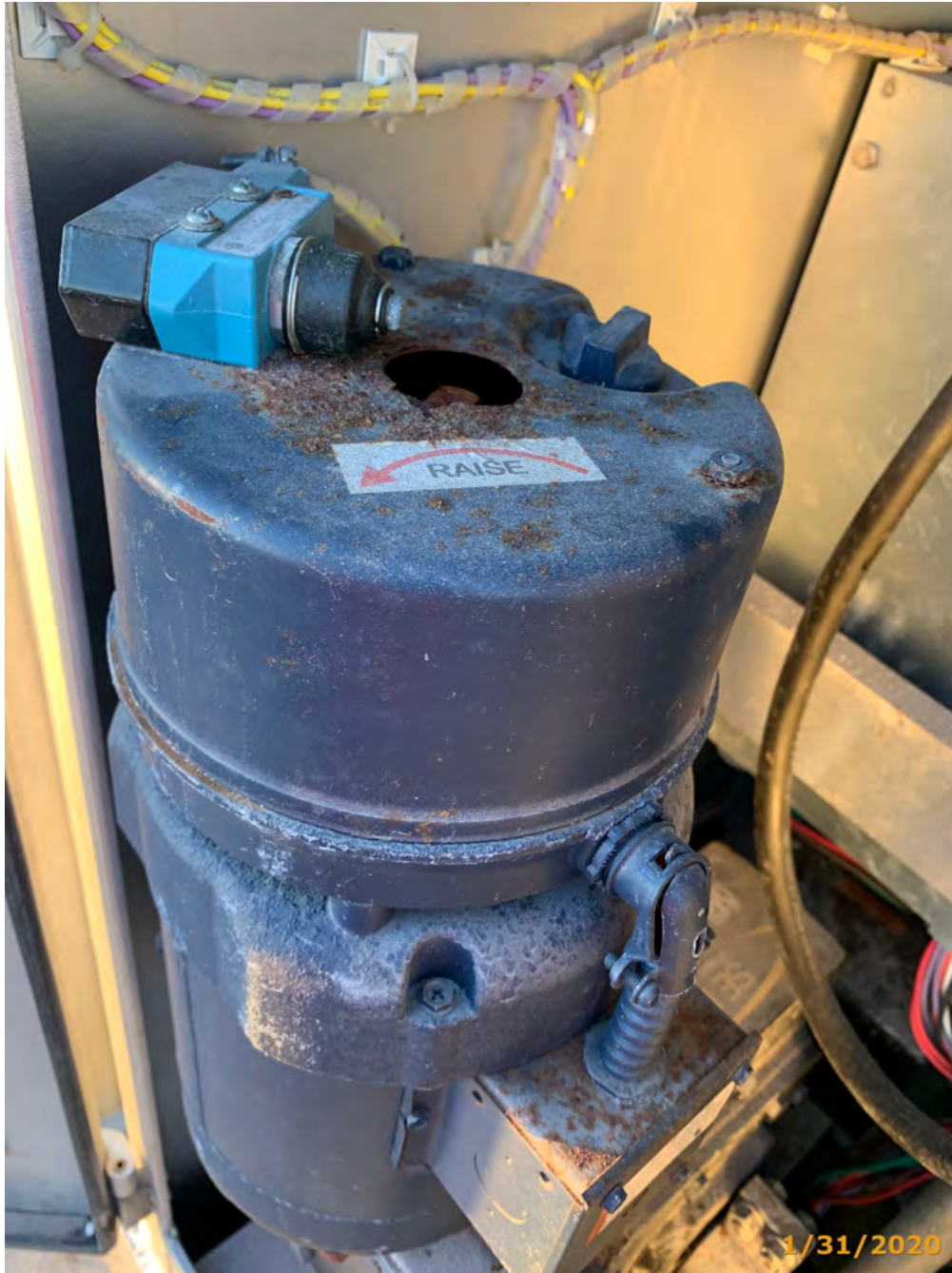
Photo 8591-E04 (Element/Env 8591/4: Warning Gates)
