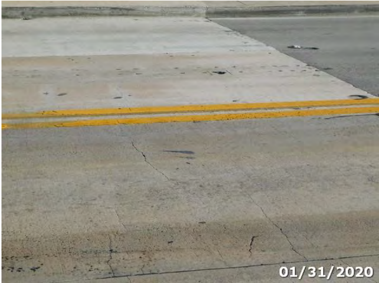
Photo 12-09 (Element/Env 12/4: Re Concrete Deck)
