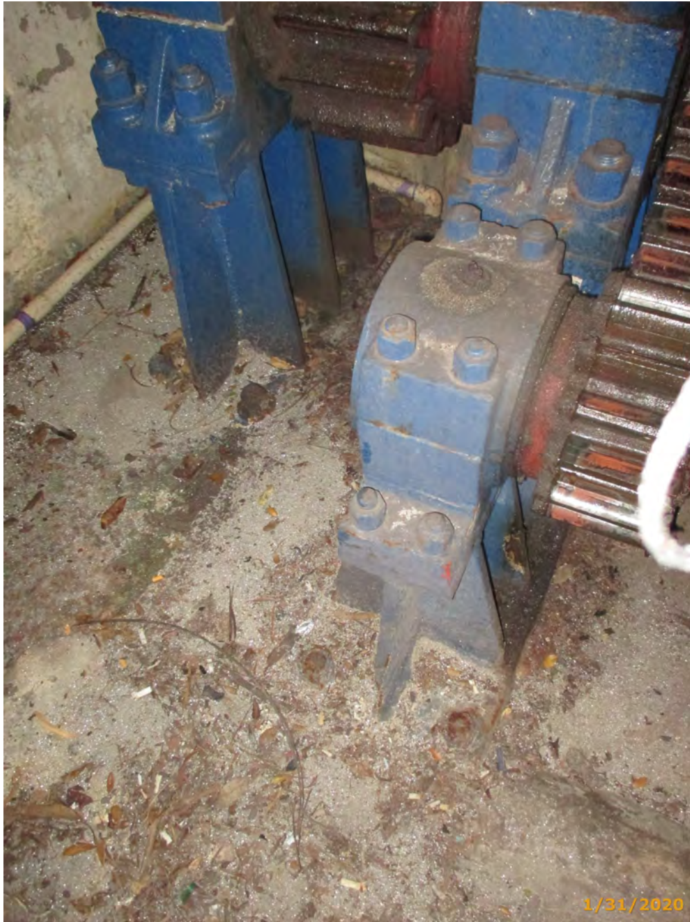
Photo 8543-M01 (Element/Env 8543/4: Shaft Bearings and Couplings)
