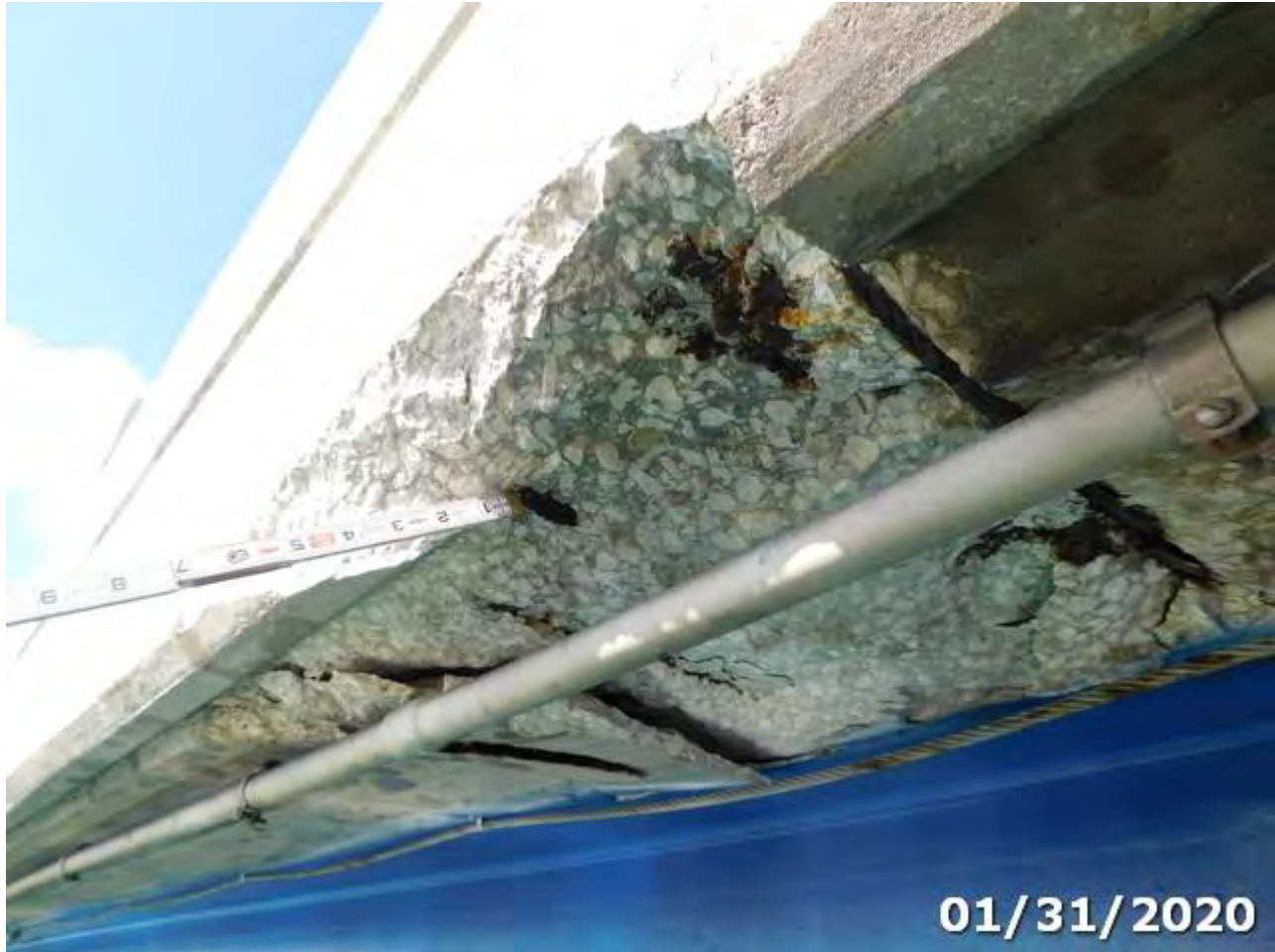
Photo 12-10 (Element/Env 12/4: Re Concrete Deck)
