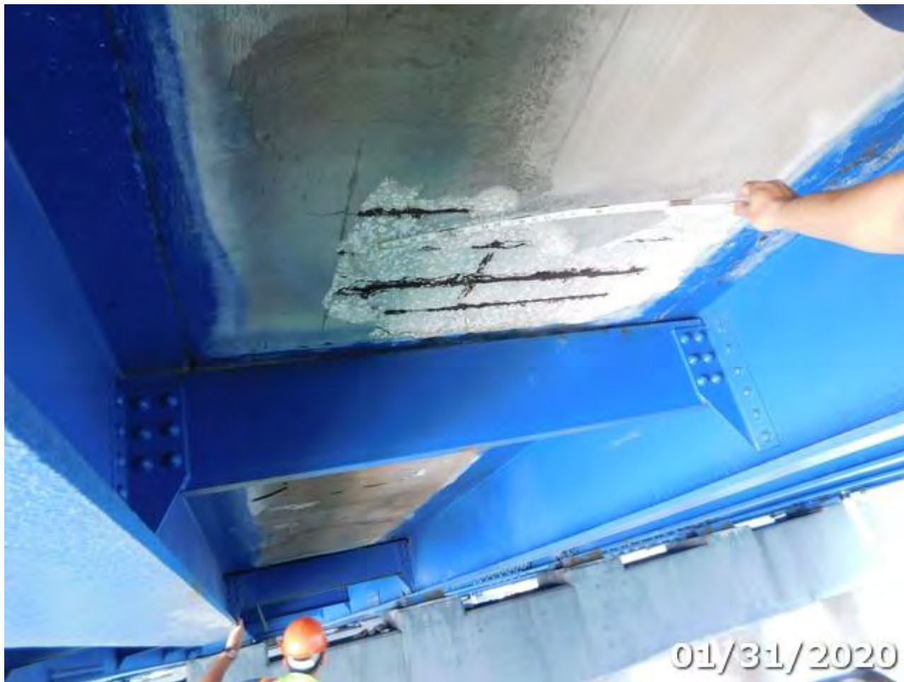
Photo 12-11 (Element/Env 12/4: Re Concrete Deck)
