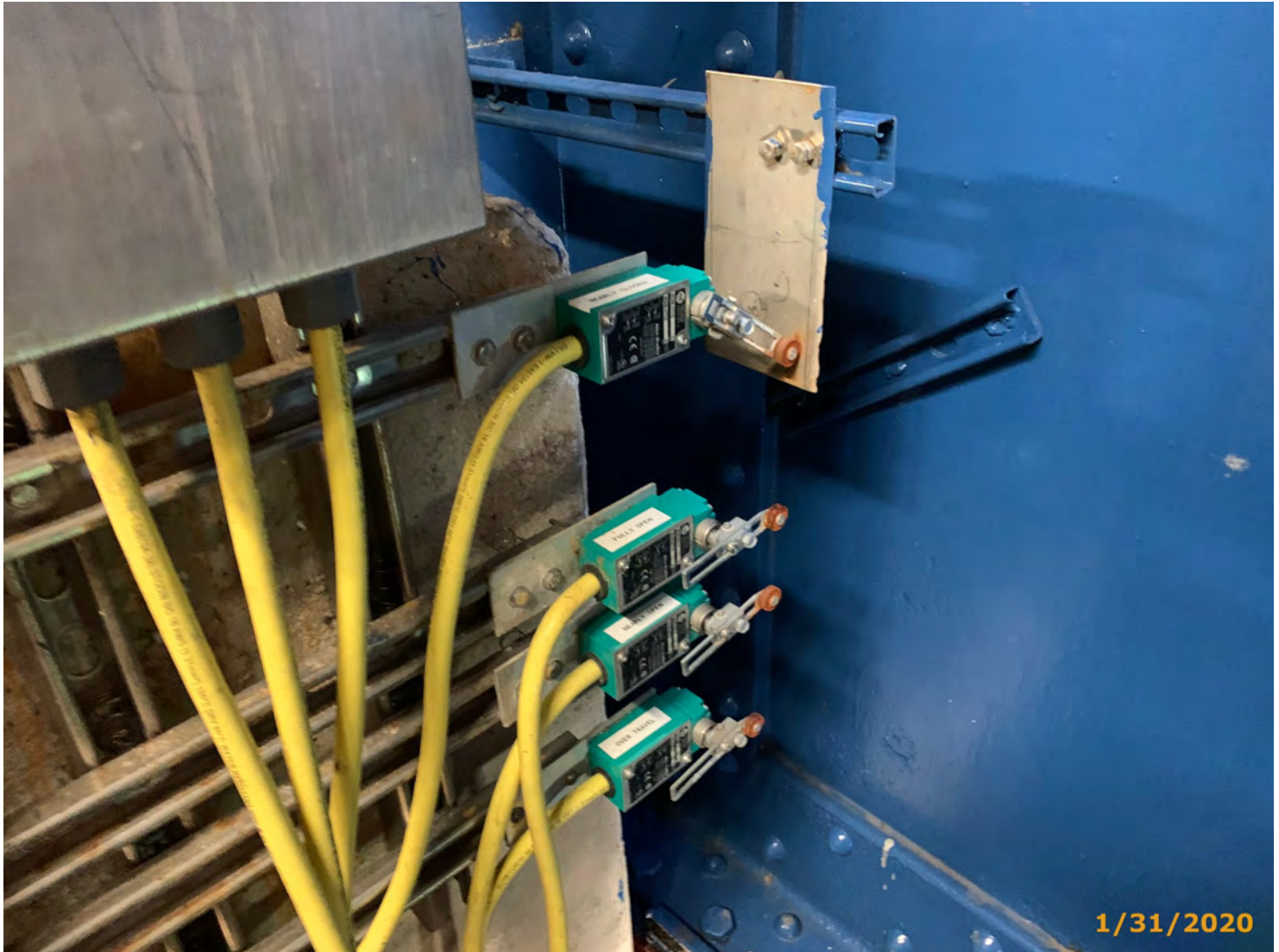
Photo 8574-E03 (Element/Env 8574/I4: Control Console)
