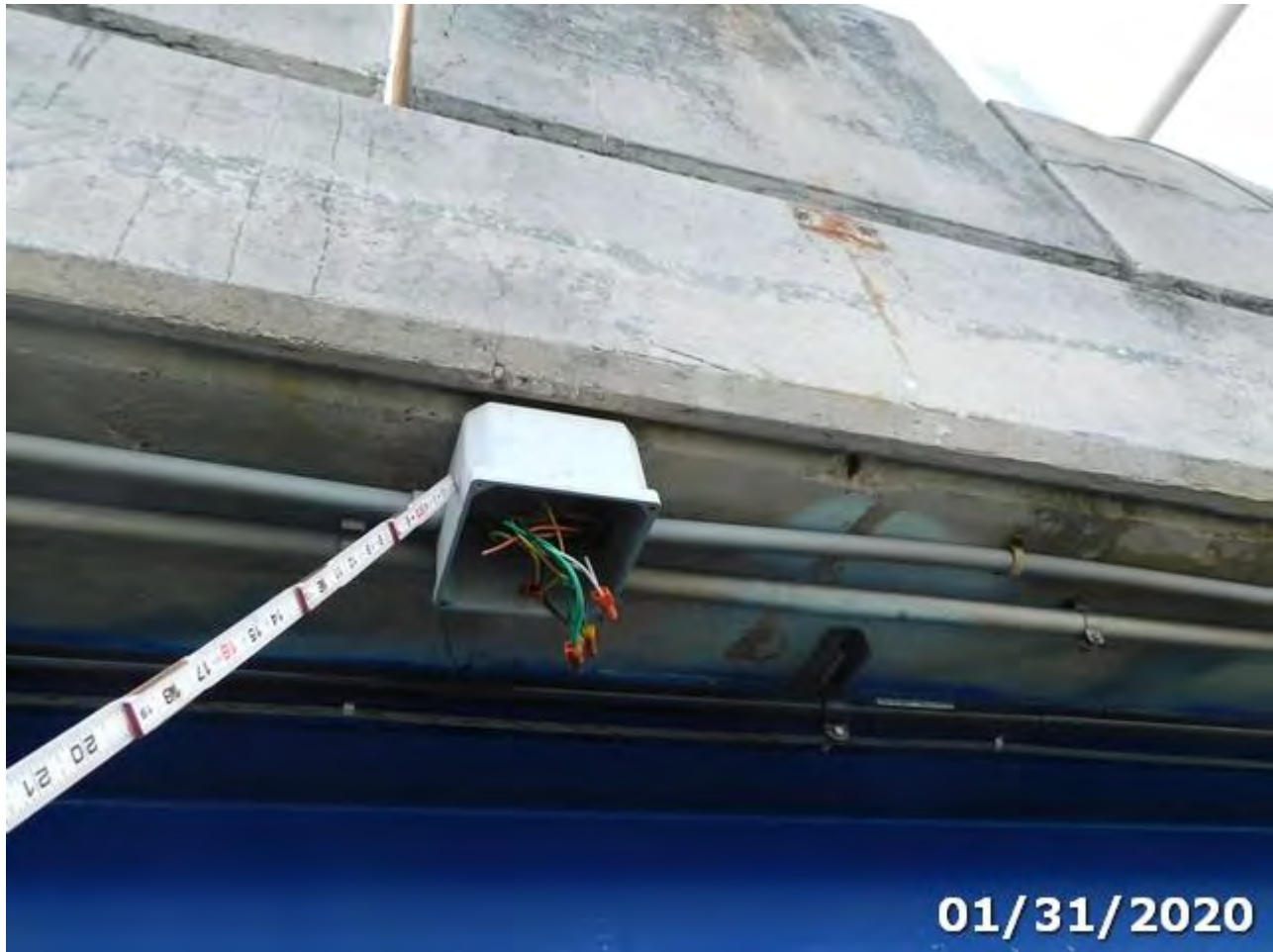
Photo 12-01 (Element/Env 12/4: Re Concrete Deck)
