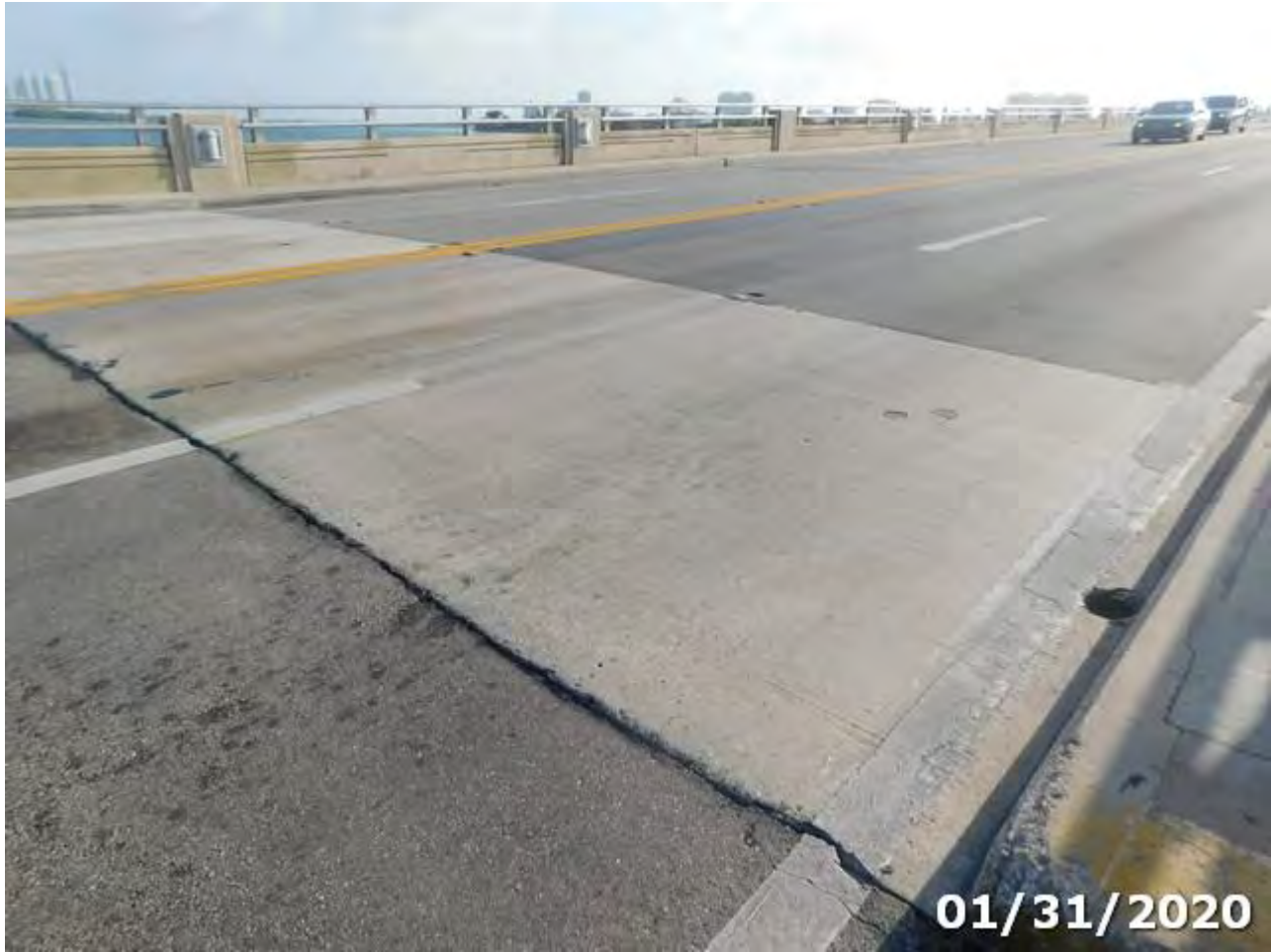
Photo 12-07 (Element/Env 12/4: Re Concrete Deck)
