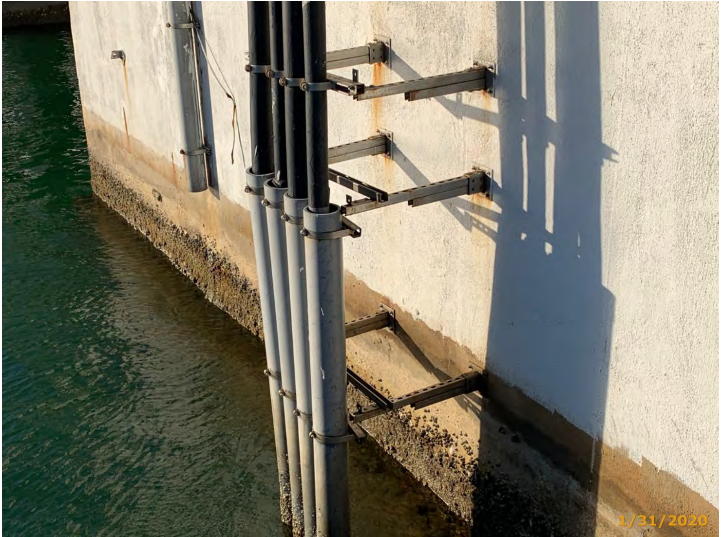
Photo 8571-E01 (Element/Env 8571/4: Submarine Cables)
