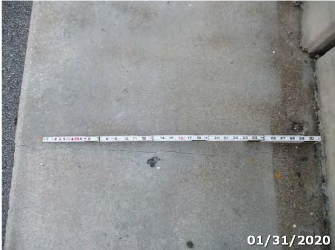
Photo 12-03 (Element/Env 12/4: Re Concrete Deck)
