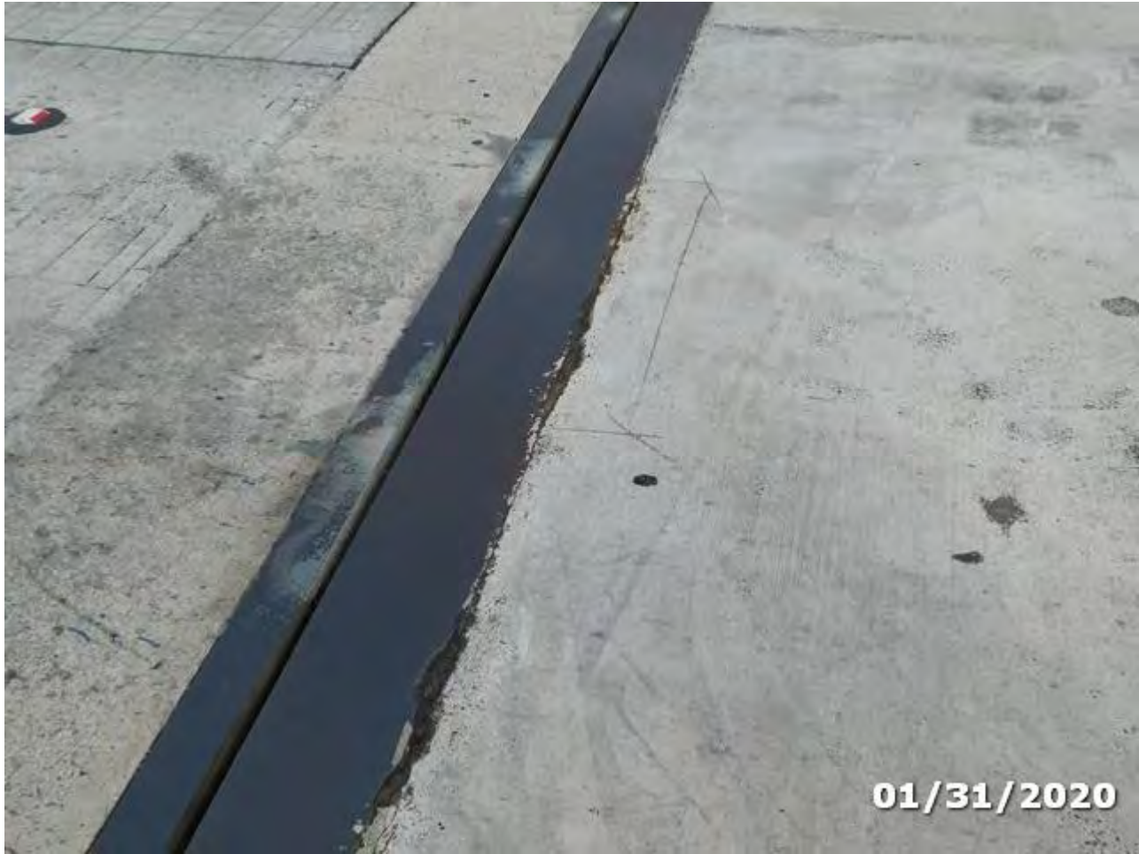
Photo 306-01 (Element/Env 306/4: Other Joint)
