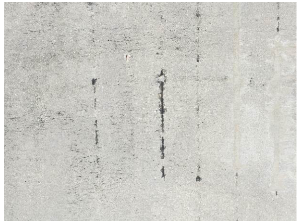
Exposed rebar at top tier slab
