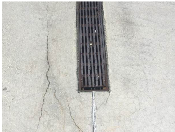
Slab cracks at top tier
