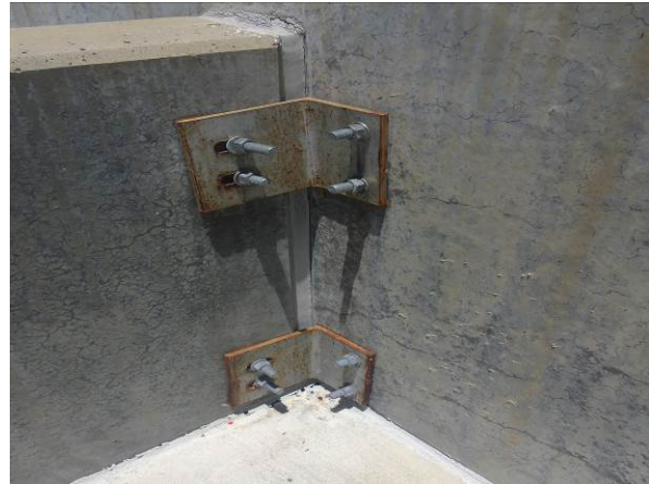
Rusted p/c connection at top tier
