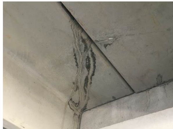
Water intrusion at failed joint sealant
