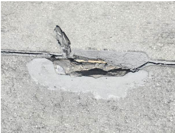
Spall at double tee connection
