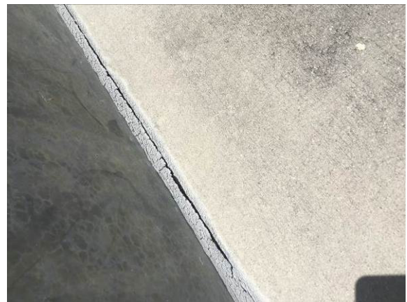
Failed core sealant at top tier
