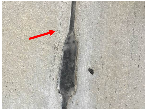
Slab crack adjacent to DT connection
