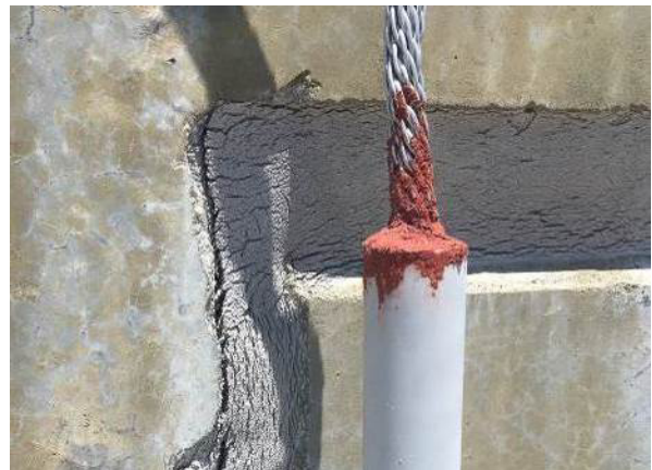
Failed vertical joint sealant
