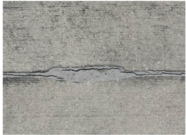
Failed joint sealant at top tier
