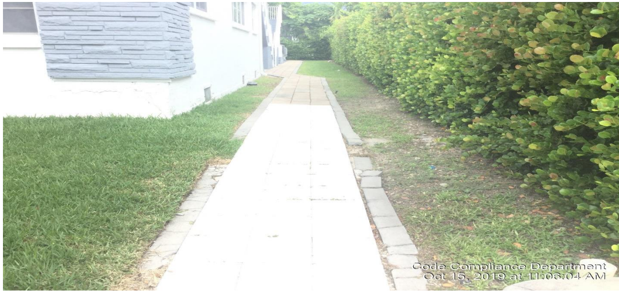
Broken brick walkway located around building 1065 98st.
