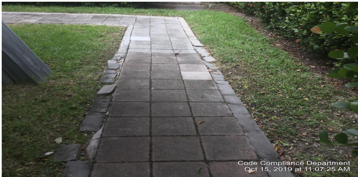
Broken brick walkway located around building 1065 98st.
