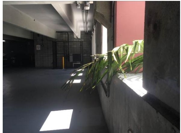
Overgrown tree branch in deck
