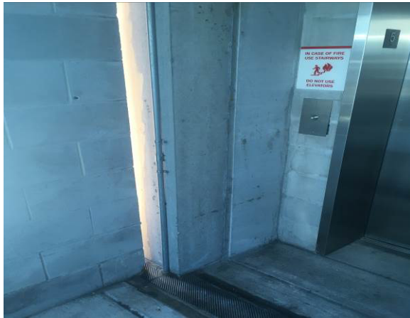
Gap at elevator lobby wall
