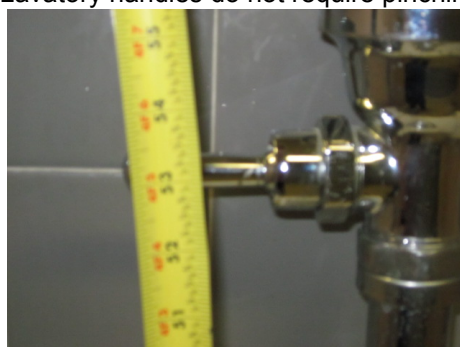
Urinal Flush valve at 53 inches
