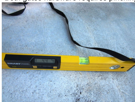
Cross slope at West gate 4.4%
