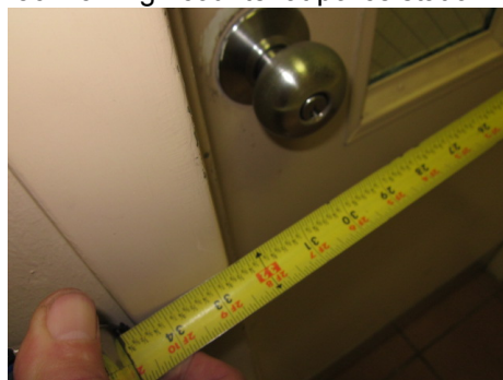
Doors provide less than 32 inches clear
