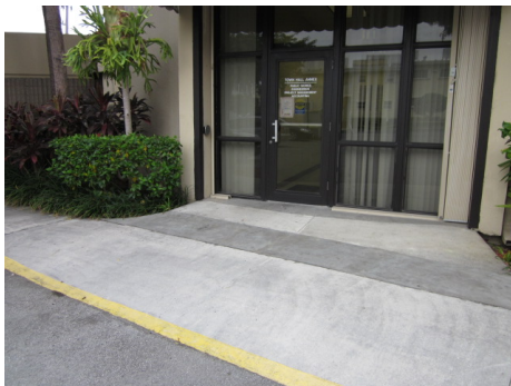
Entrance door has low power opener
