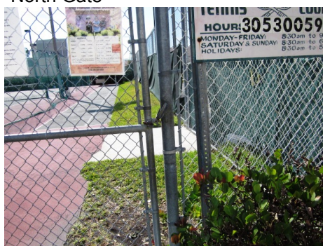
Both gates hardware requires pinching
