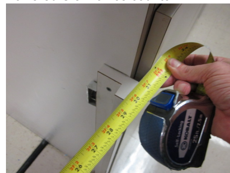
Gate to office area less than 32 inches
