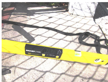
North gate ramp running slope 20.1%
