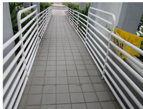
Railing not continuous
