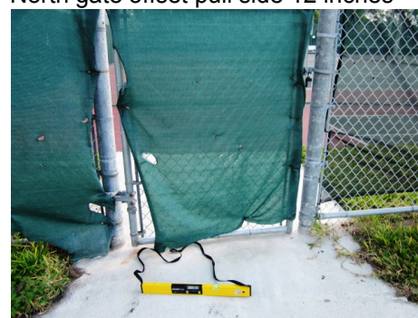
Cross slope at West gate 4.4%
