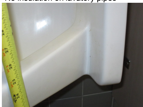
Urinal lip at 25 inches above floor
