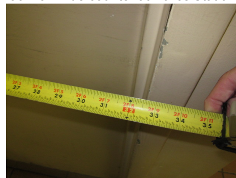
Doors provide less than 32 inches clear
