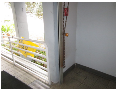
Ramp railing with no extension
