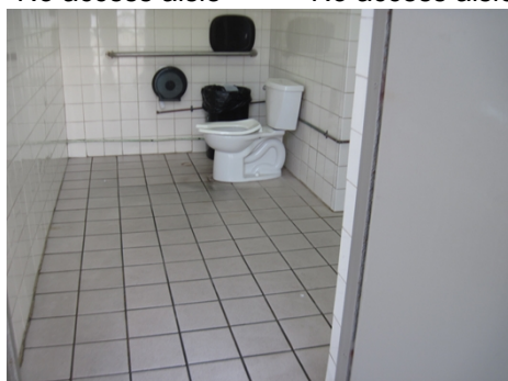
Toilet paper dispenser needs relocation
