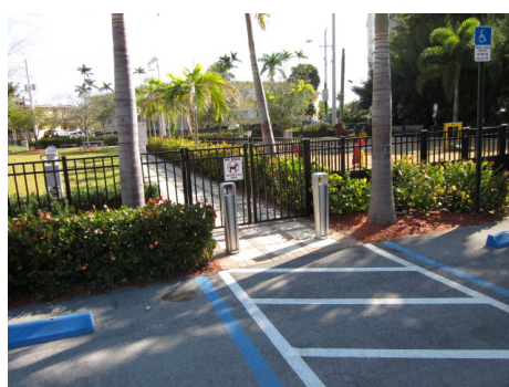
North gate ramp running slope 20.1%
