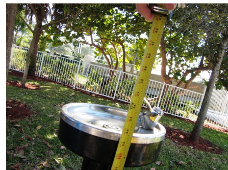
No high drinking fountain
