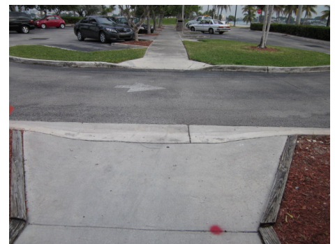
Ramp landing not level
