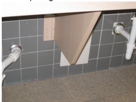
No insulation on lavatory pipes
