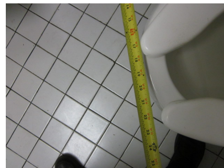
Toilet to side wall not 18 inches
