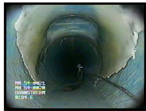
Fig 7. Delaminated Lateral Liner
