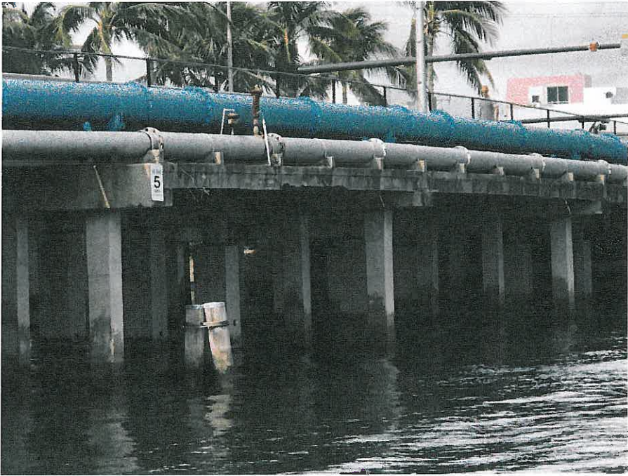
DAMAGED SUPPORT SPAN ON NORTH SIDE OF BRIDGE
