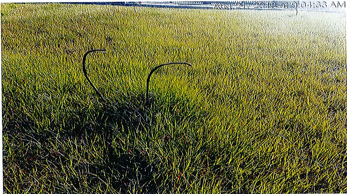
Found rebar protruding from the ground.
