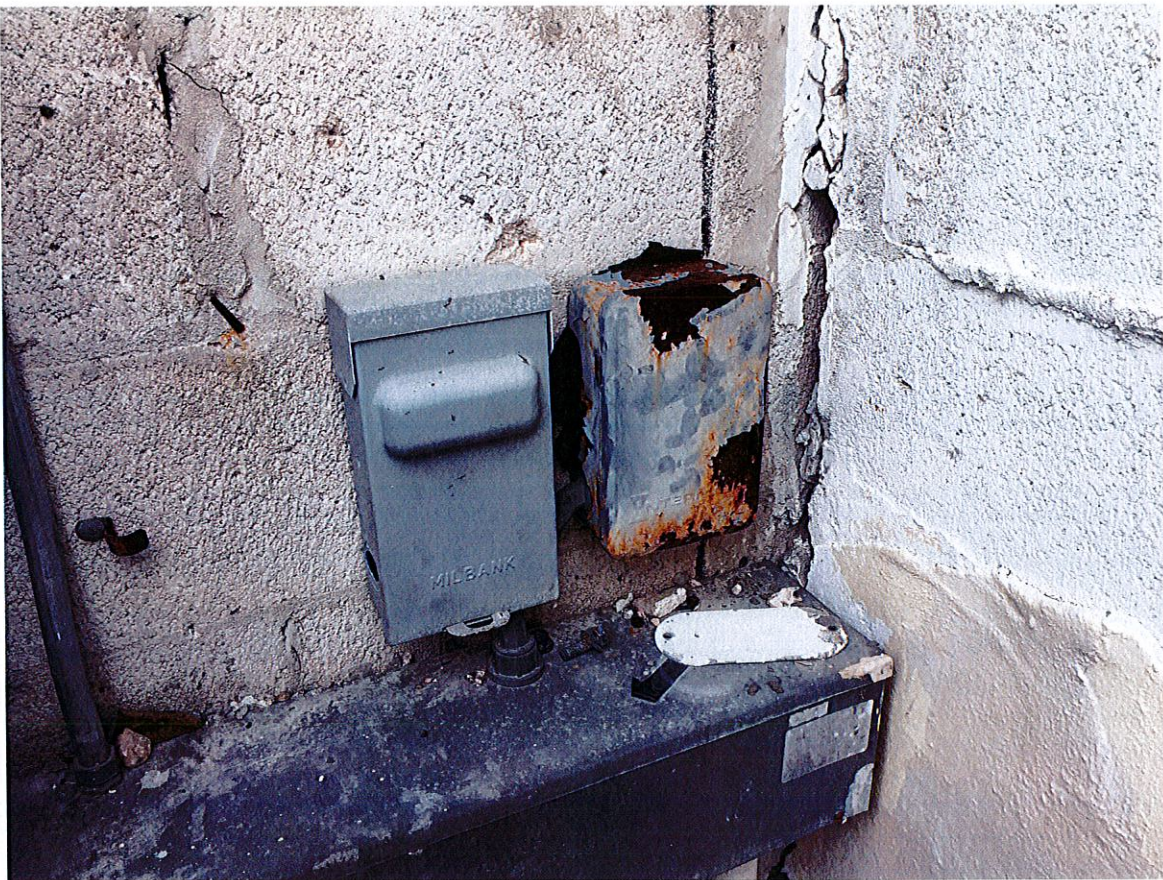
9725Electrical3.JPG Electrical Inspection TDR May 03, 2018
