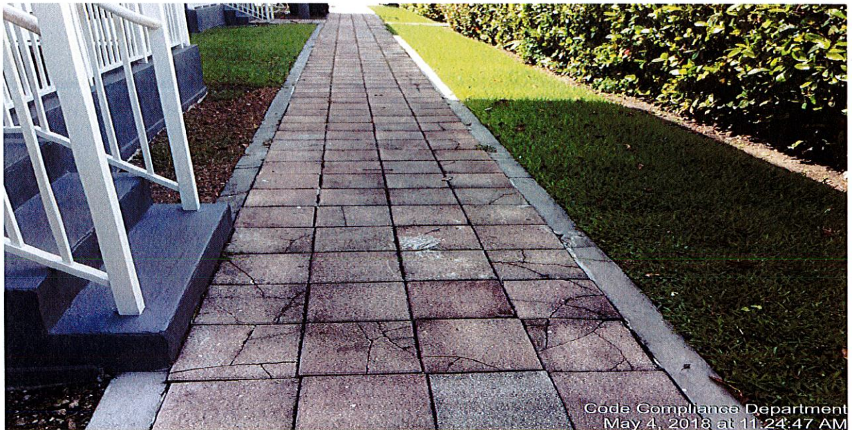
Broken brick walkway located around building 1065 98st.
