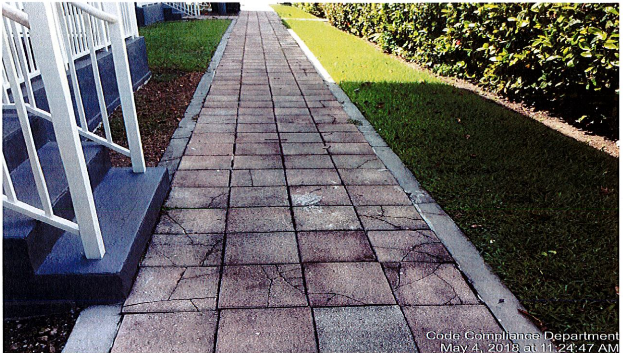
Broken brick walkway located around building 1065 98st.
