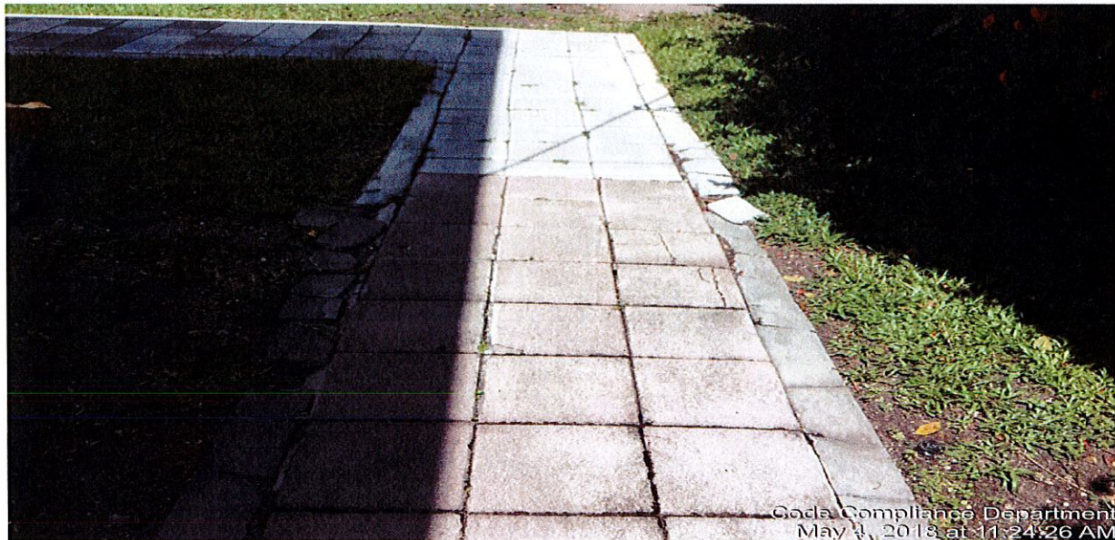
Broken brick walkway located around building 1065 98st.
