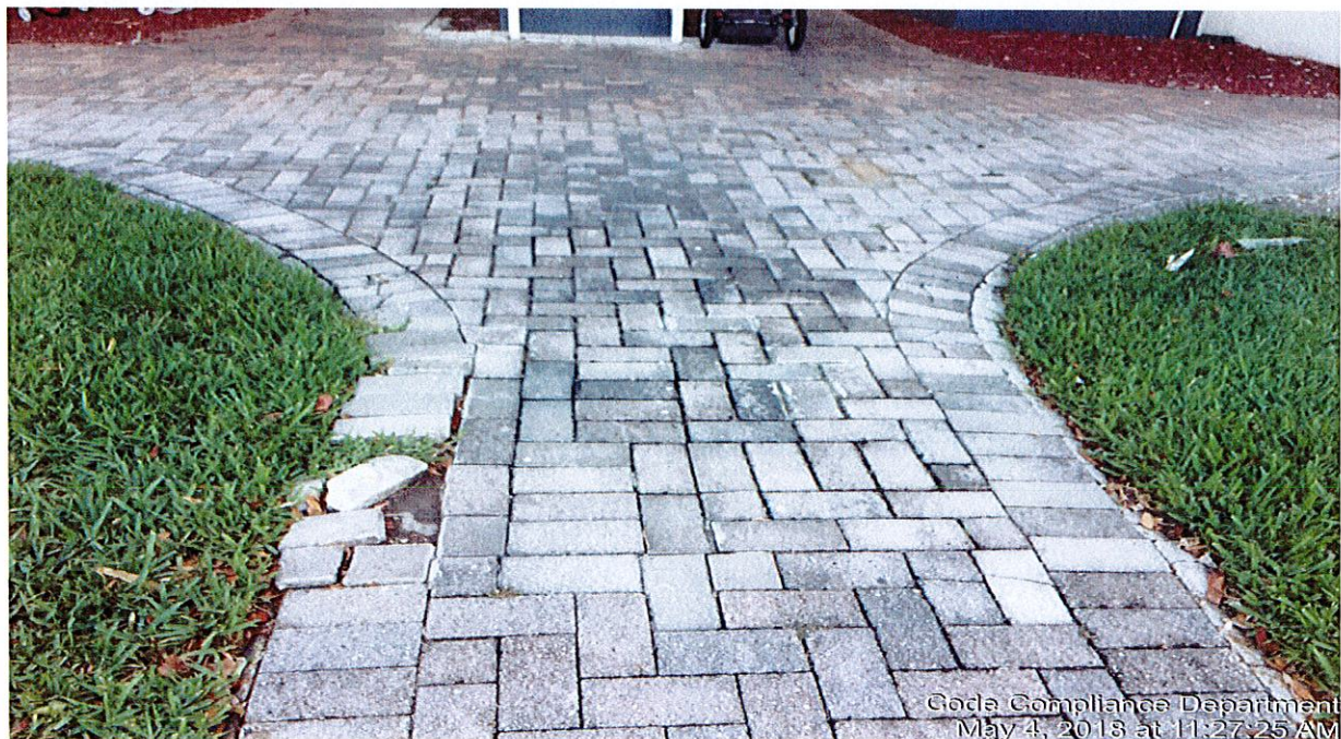
Broken brick pavers located at the building entrance.
