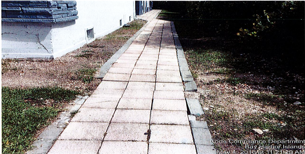
Broken brick walkway located around building 1065 98st.
