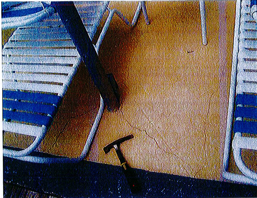
Photo 599: Property 147 – Settlement cracks on pool deck.
