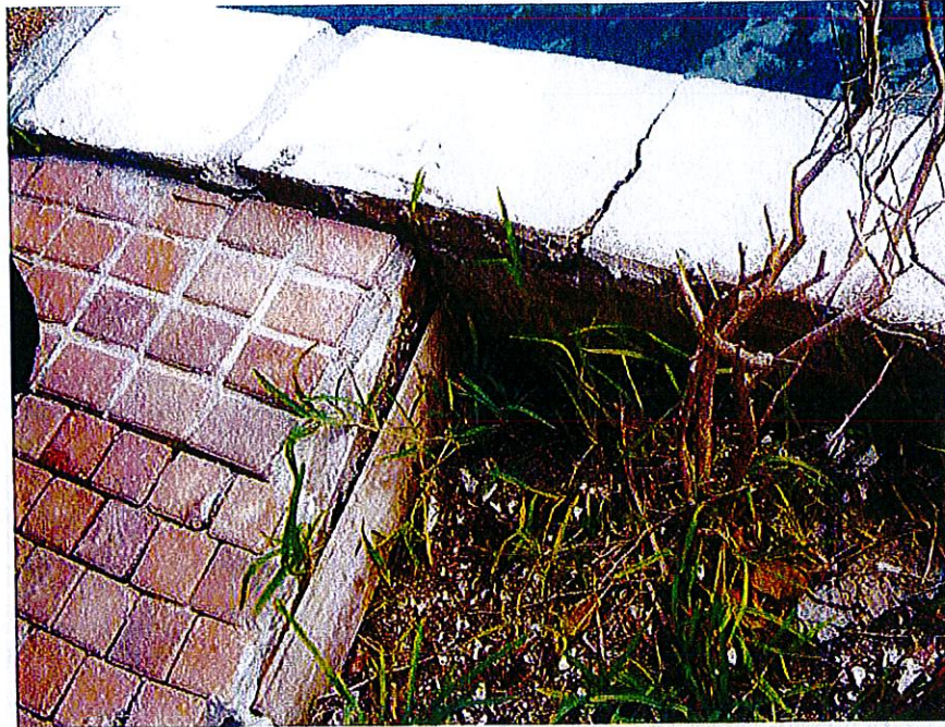
Photo 601: Property 147 – Brick walkway behind spalled cap is settling. There is also a hole approximately 18" deep at the location.
