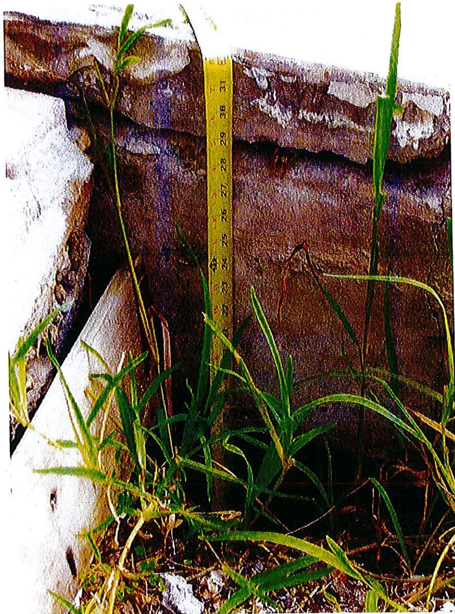
Photo 602: Property 147 – Close-up of 18" deep hole under brick walkway area.
