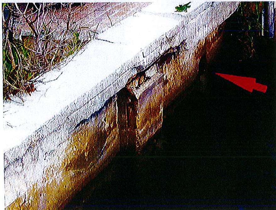
Photo 600: Property 147 – Concrete spall 8 LF in length east of dock. Also note pipe outfall (arrow).
