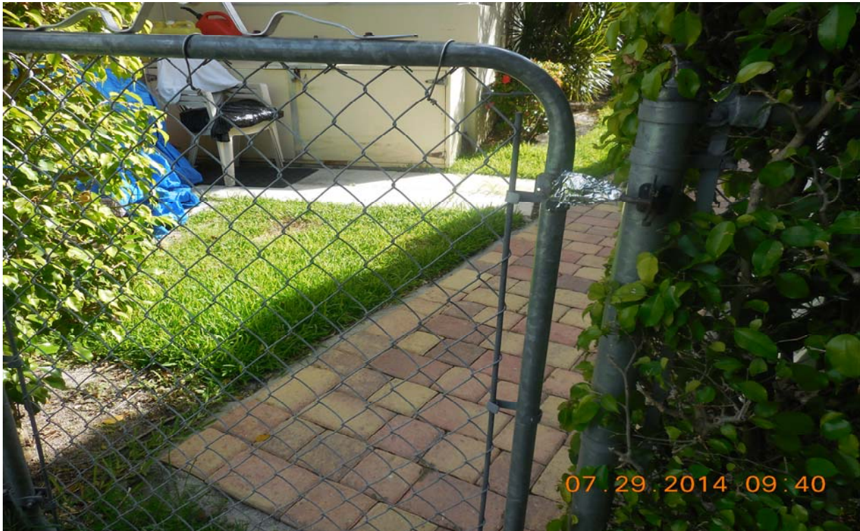
Southside pool gate is in disrepair.
