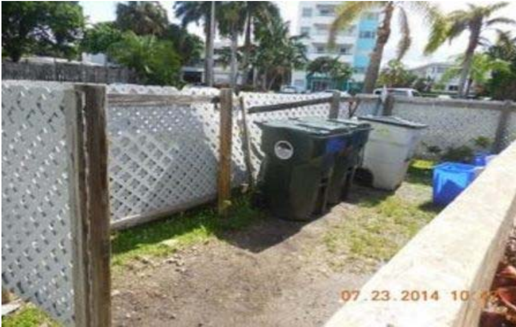
Garbage enclosure facing 98 street is in disrepair.
