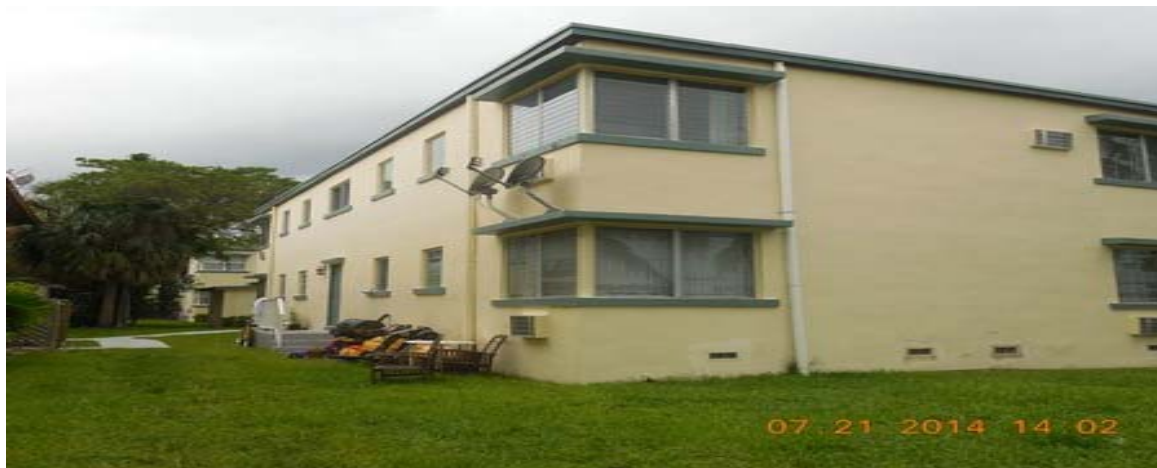
Building 10270 – No exterior lighting provided.
